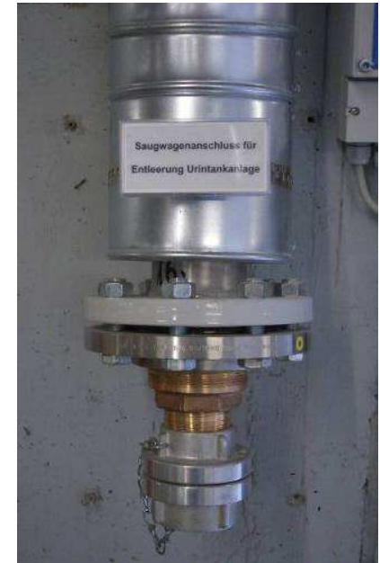
Docking station for vacuum tanker
