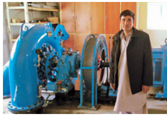
Electricity from hydropower / Badakhshan Province
