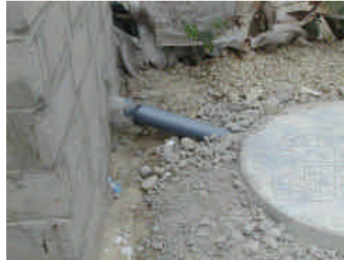
Figure 4: A short tube connects the latrine to an off set pit, which later can be connected to a small-bore sewer.
