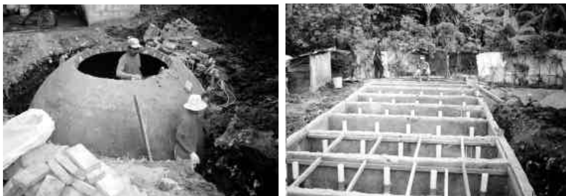
Figure 2: Biogas Digester (left) for part-stream treatment of "blackwater", brick construction with waterproof airtight plastering. Baffled reactor (right), based on anaerobic up-flow principles.
