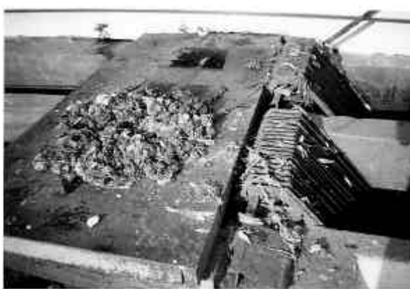
Figure 3: Screens out for sewer, source: field data 2002
