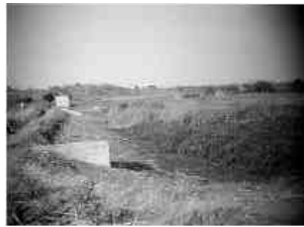
Figure 5: Dilapidated manhole, source: field data 2002
