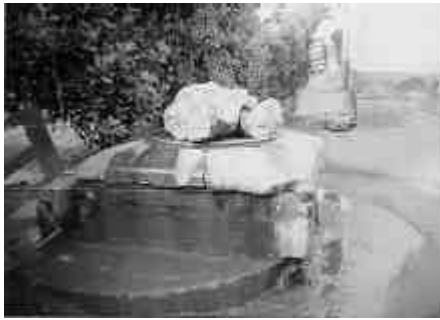
Figure 4: Dilapidated manhole, source: field data 2002
