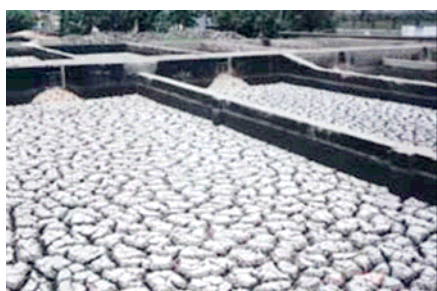
Figure 2: Large lumps in overfilled drying beds (source: ipp consult)
