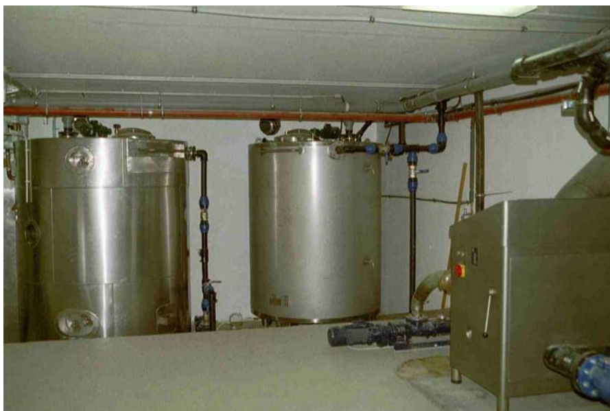
Figure 6: Mixing and hygienisation unit (source: Otterwasser) kitchen and bathroom) is transported by gravity pipes to several constructed
