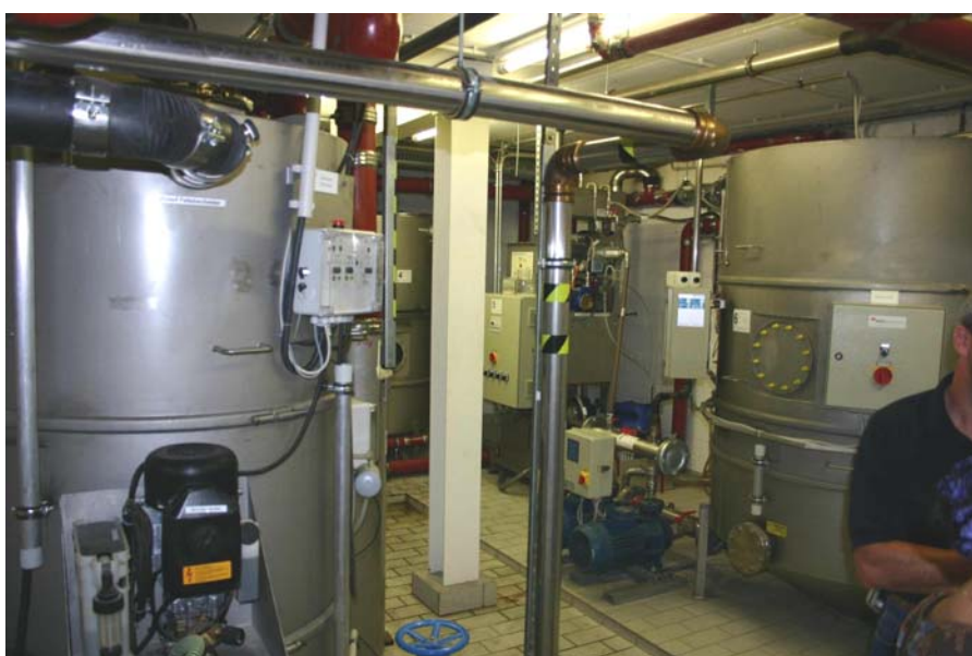
Figure 4: Greywater treatment facility in KfW Ostarkade (Photo: GTZ)
