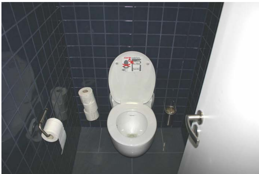
Figure 2: Vacuum toilet in KfW building Ostarkade (Photo: GTZ)
