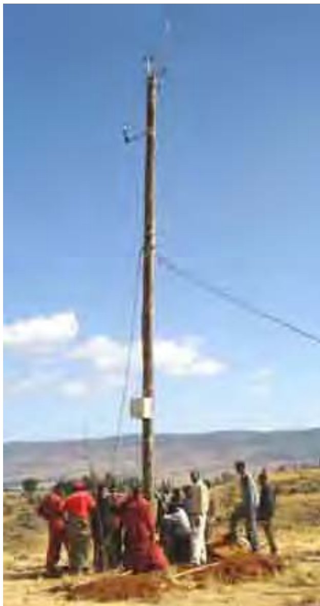
Figure 1-11: 10 m Tower with Anemometer, Wind Vane and Lightning Arrestor (Sululta)
