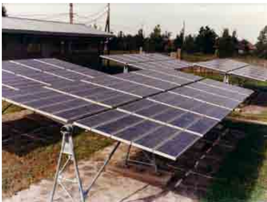
Figure 2-5: Village Grid System by Photovoltaics – Mita with 31.5 kW
