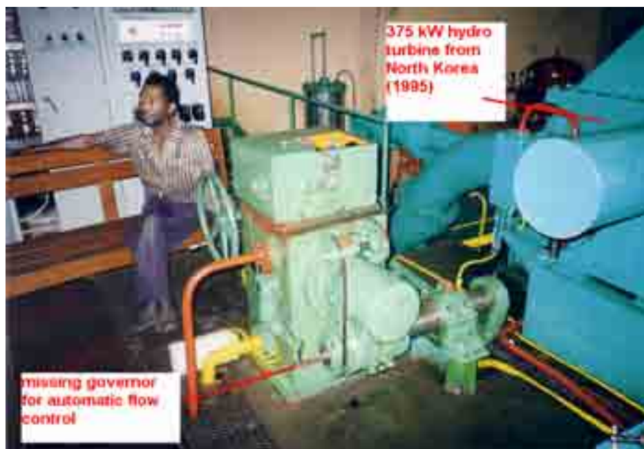
Figure 5-3: Manually controlling a 375 kW Water Turbine
