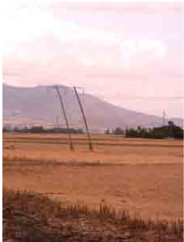
Figure 5-2: 66 kV Overhead Line (between Woliso and Addis Ababa)
