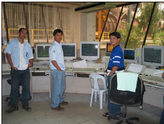
The control room of the cement plant
