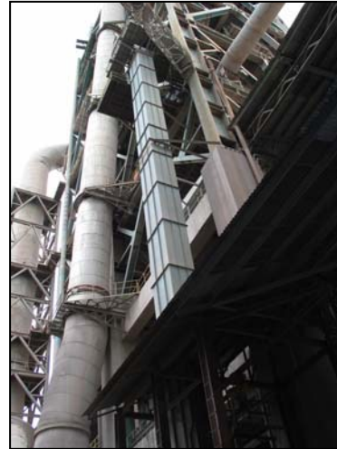
The conveyer runs in the angular tunnel
