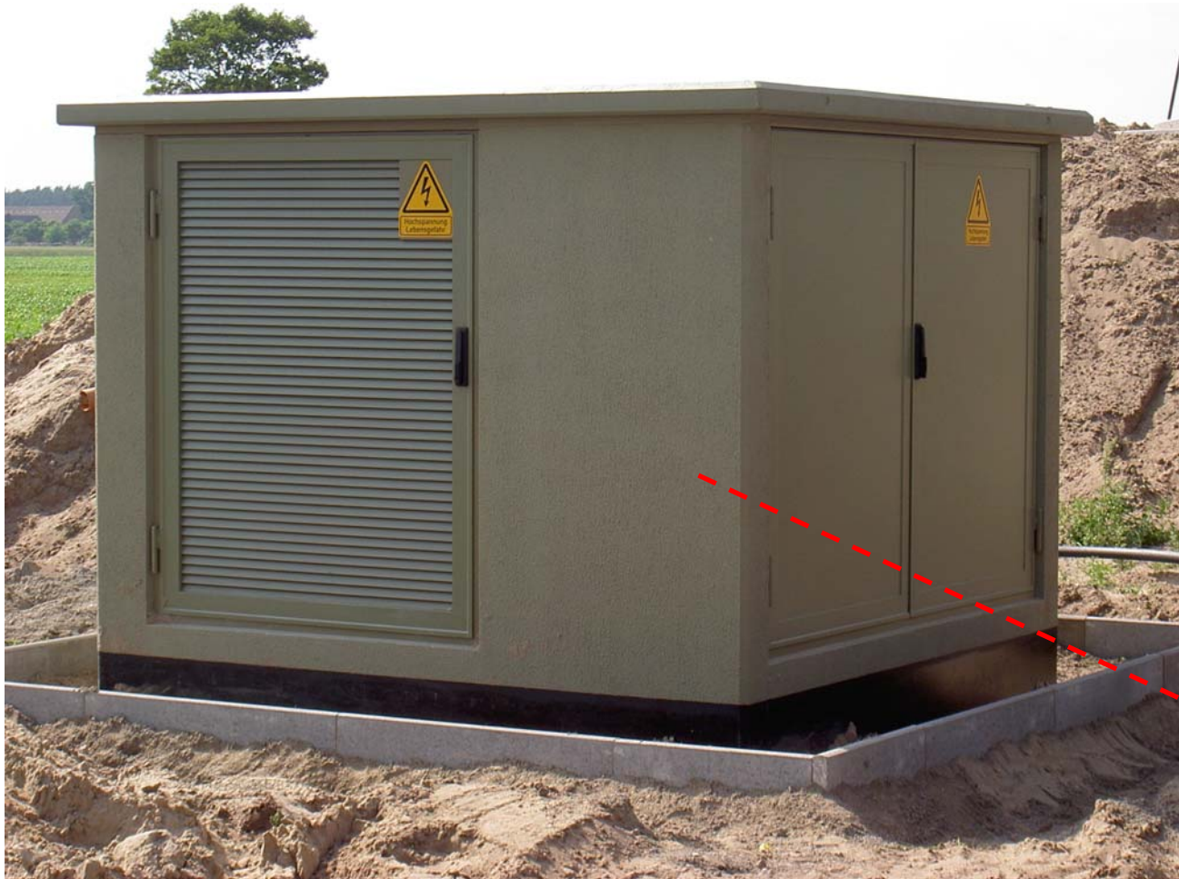
Transformer 690V/20kV, 1.8 MVA
